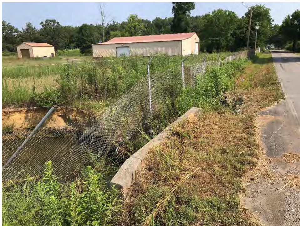
Drainage feature on Shellmound Rd
